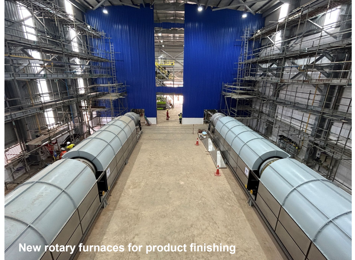
New rotary furnaces installed to increase Product Finishing efficiency
