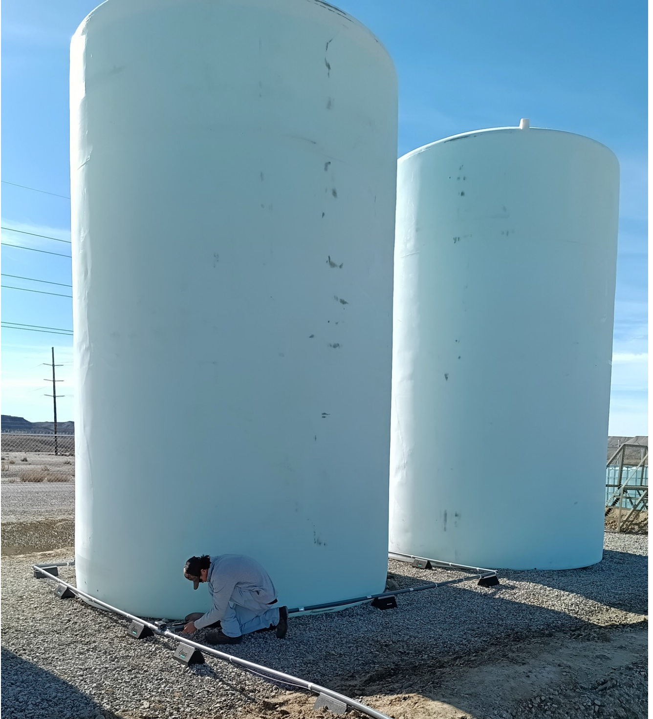
Figure 4: Two full tanks containing 32,000 gallons of lithium eluate processed by the Koch DLE at Green River, Utah, USA
